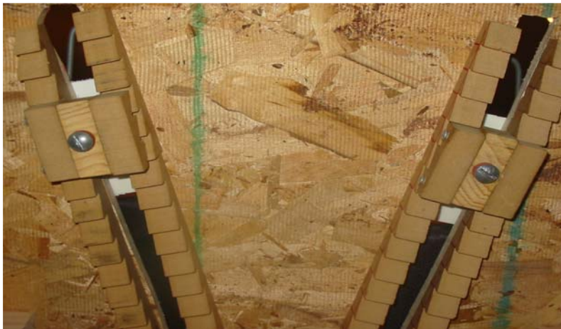
Figure 8: Strap Anchor of Prototype (Back View)
